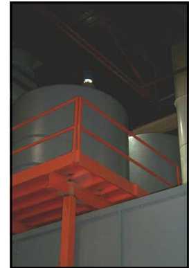
2 2500 gallon plastic R.O water tanks give ACL lots of capacity & flexibility.
