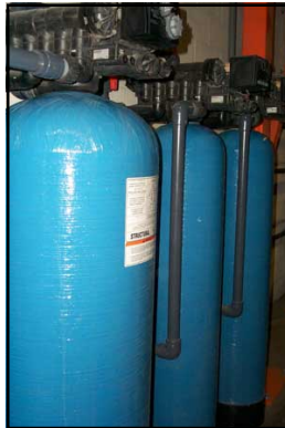
The ultra clean water is actually corrosive to mild steel. Everything must be built from plastic, stainless steel or epoxy coated steel.
