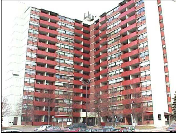
This building is subjected to north, south, east & west exposure. Standing up perfect through 2 harsh winters.
