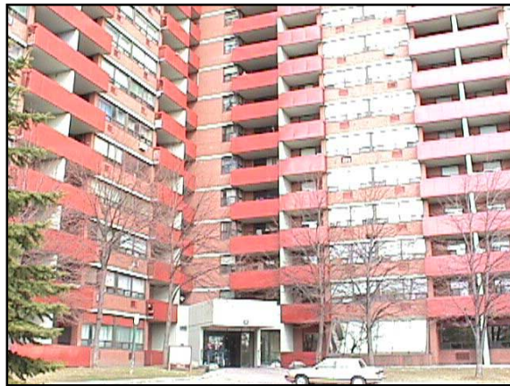
This property management firm found recoating existing panels cost effective and are considering the same on future upgrades.
