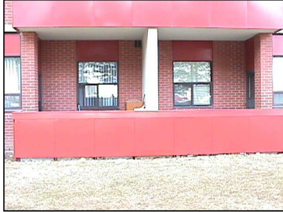
The coating shows no damage or degradation even at ground level where weekly greenskeeping or snow removal takes place.
